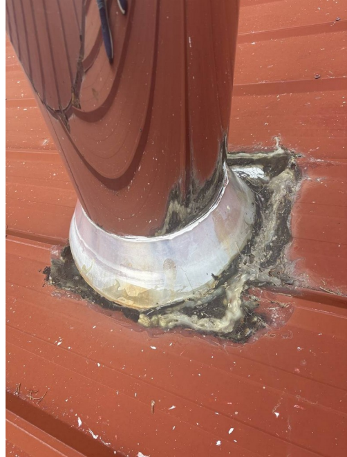
4 Chimney jack. Old mastic cracked and pulled back.
