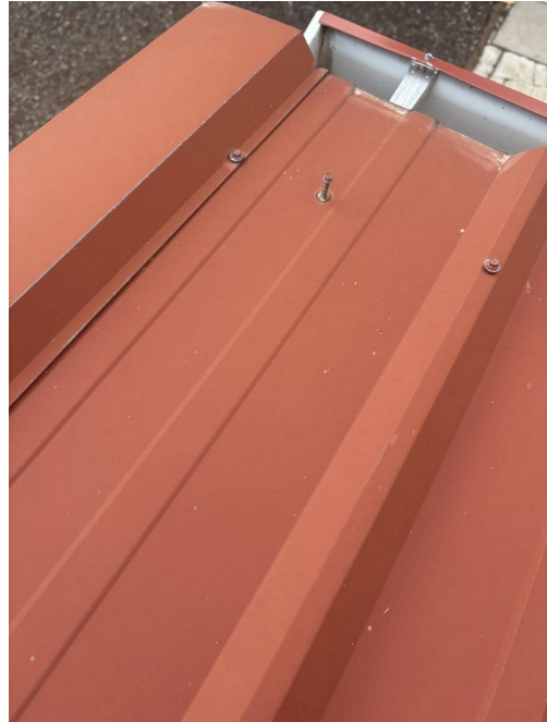
6 Screw standing up near the eave. Threads showing. Washer not tight.
