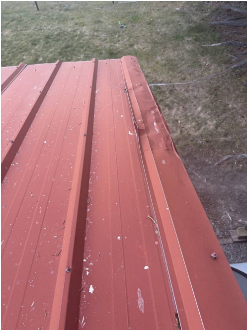
10 Gap down the rake. Water can get behind the metal onto the fascia.
