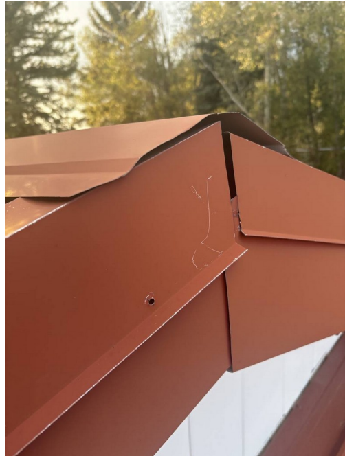
11 Corner of the trim. Pieces do not meet. Empty screw hole.
