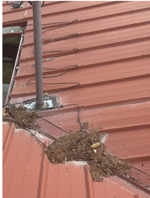
15 Mast through a patch. Cables across the ribs into a dirty valley.
