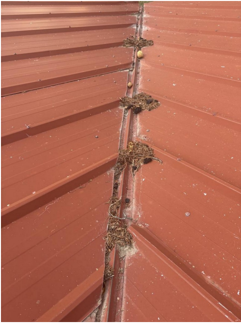
12 Valley. Poor cut. Needles, cones, and sticks in the waterway.
