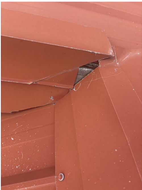
1 Garage corner. Metal does not meet. Wood in the hole.
