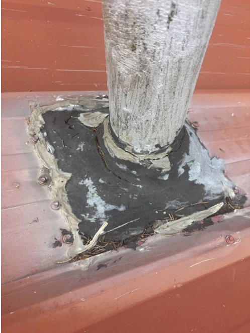
3 One of three vents. Asphalt sheet and mastic. Peeling. Needles under the edge.
