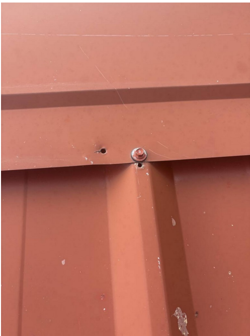
7 Empty hole next to a screw, and another hole at the rib.
