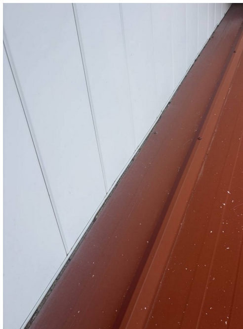
2 Roof run to the white wall. No step flashing. No wall trim.
